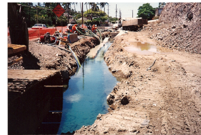
When the DOT widened the highway, flows from the spring were somehow obstructed and fresh spring water flooded the DOT construction project. Source: Maunalua Fishpond Heritage Center
