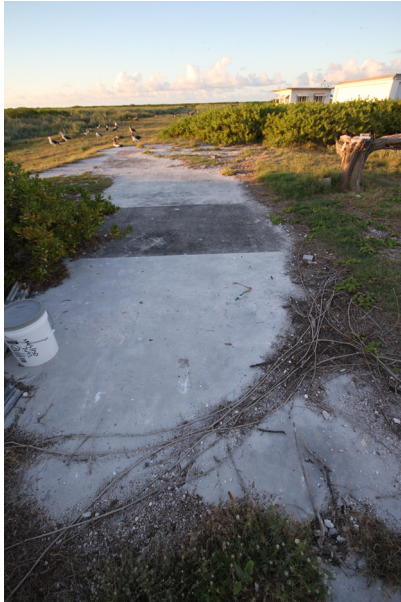
The existing slab on the site was repurposed for use as a bunkhouse. (Source: DOFAW)
