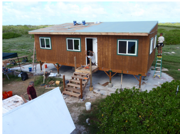
A view of the front of the new bunkhouse under construction. (Source: Kure Atoll Seabird Sanctuary)
