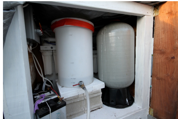
Reverse Osmosis Water System
