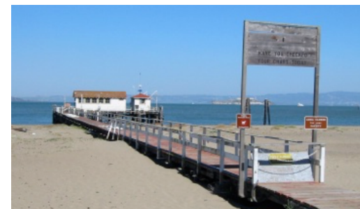
Pier on San Francisco Bay Currently deteriorated and closed. Funded for rehabilitation. Crissy Field, San Francisco, CA
