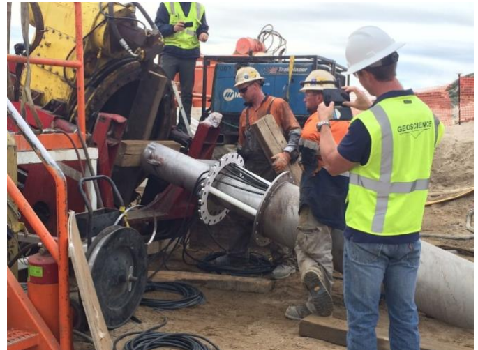
A California American Water Company test well is installed. Photo: Bridget Hoover/NOAA
