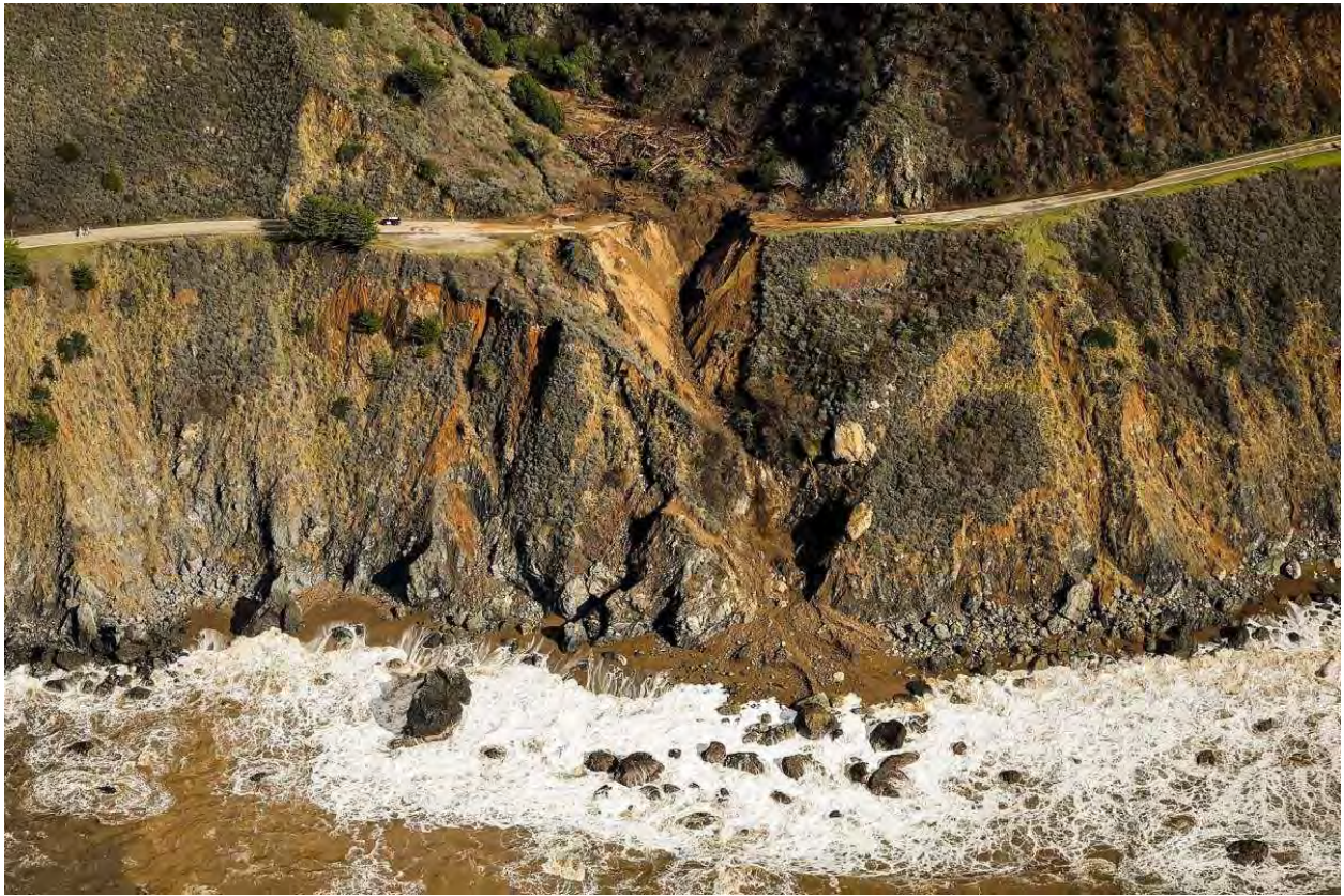
Rat Creek slide along Highway 1 in Big Sur occurred in January 2021. Photo: Gabrielle Lurie/San Francisco Chronicle
